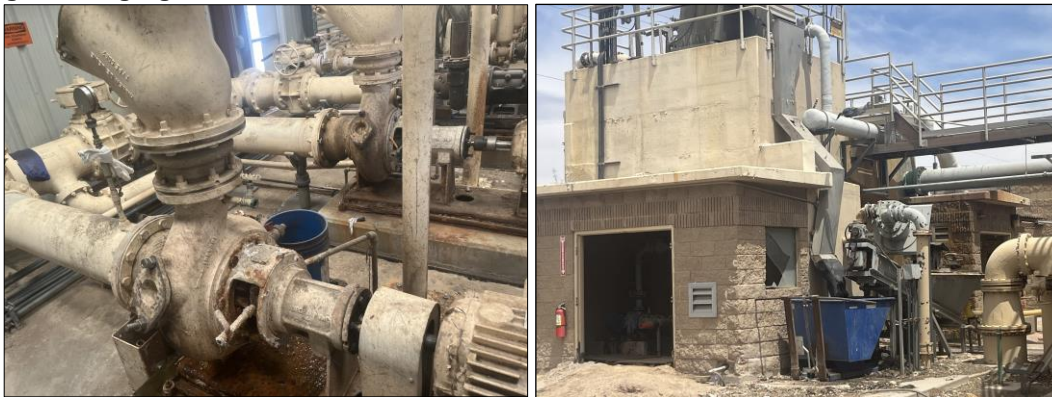
Figure 5. Aging Water Infrastructure at CRRUA Sunland Park Arsenic Treatment Facility
