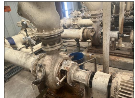
Figure 1. Aging Water Infrastructure in Sunland Park
