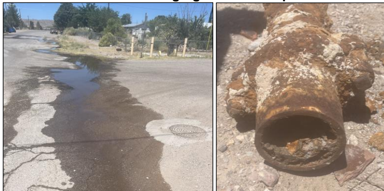
Figure 6. Water Loss in the City of Truth or Consequences Because of Aging Waterline Pipes
